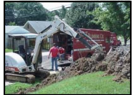
St. Louis County's Sewer Lateral Repair Program pays for hundreds of major repair jobs like this every year.
